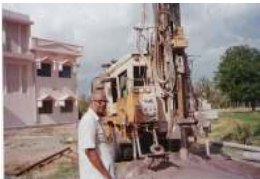
Bore well at St. Xavier's Seminary, 2000
